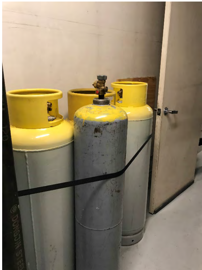
Photograph 30: View of 407C refrigerant cylinders.
