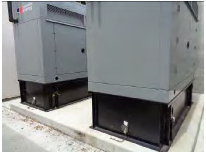
16. View of back-up generators
