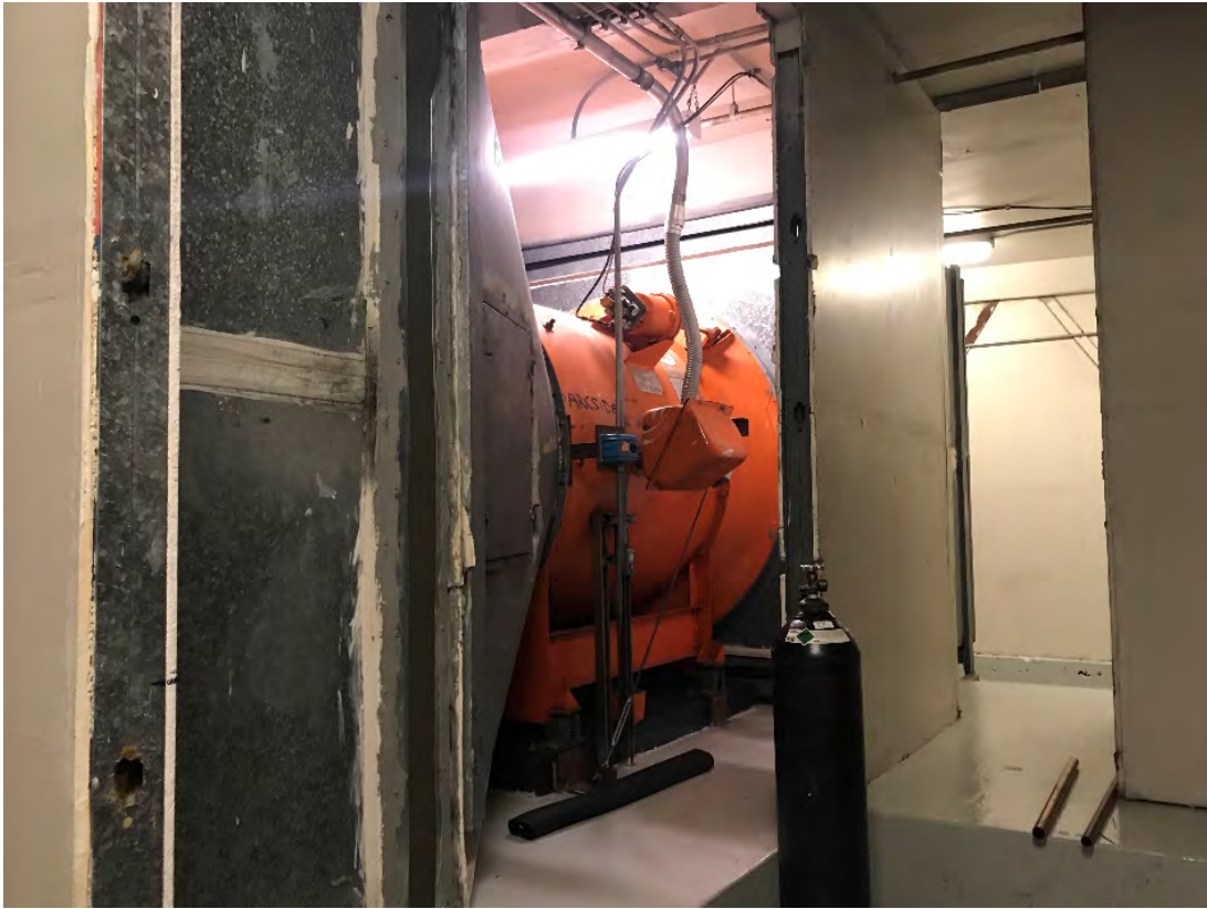
Photograph 29: View of joy fan located on the roof of the Property.
