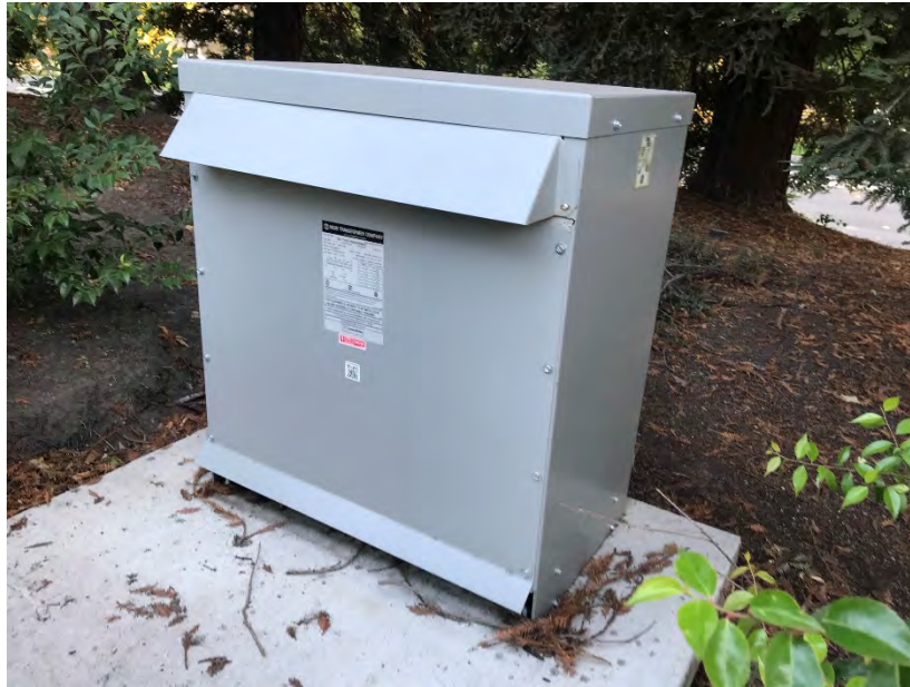
Photograph 5: Example of transformer located along the eastern boundary of the Property.
