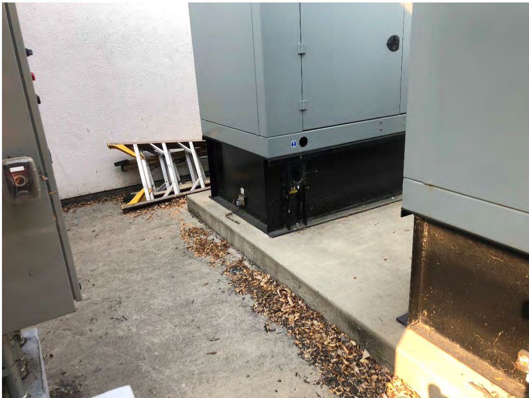
Photograph 8: Backup generator machinery. No staining observed.
