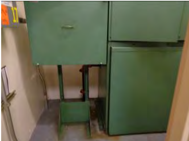
39. View of elevator equipment for Building 2430
