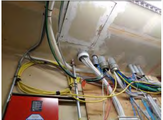
44. Telephone Equipment Room – Building 2440
