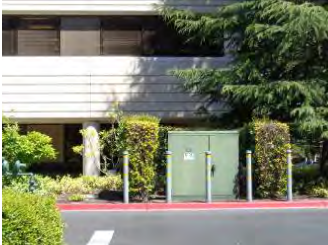
19. View of transformer
