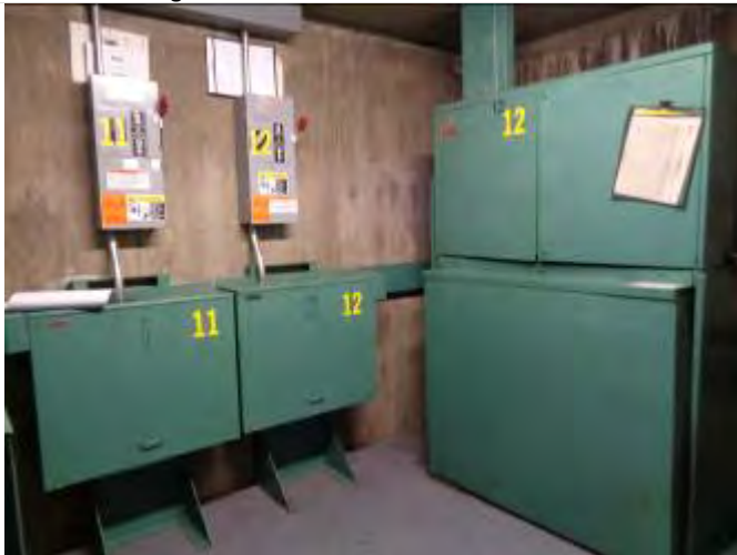
27. View of elevator equipment for Buildings 2400-2410
