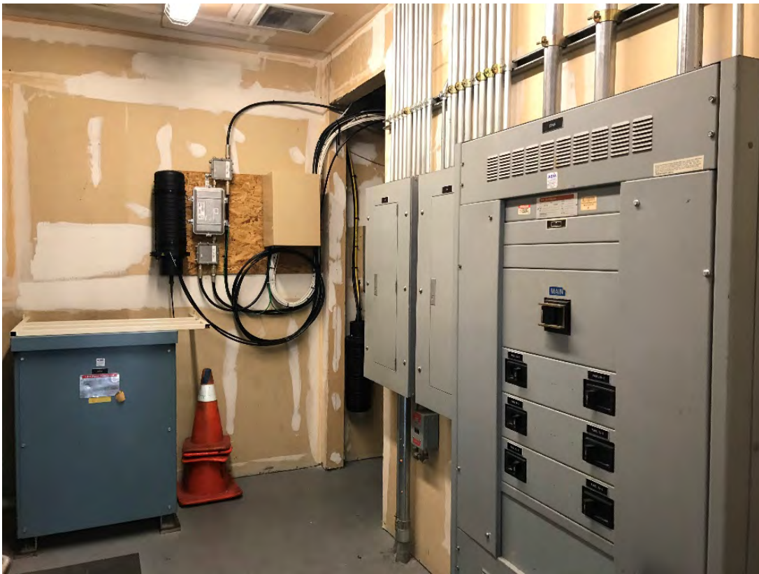
Photograph 26: View of the other side of a typical electrical control room located in the Property.
