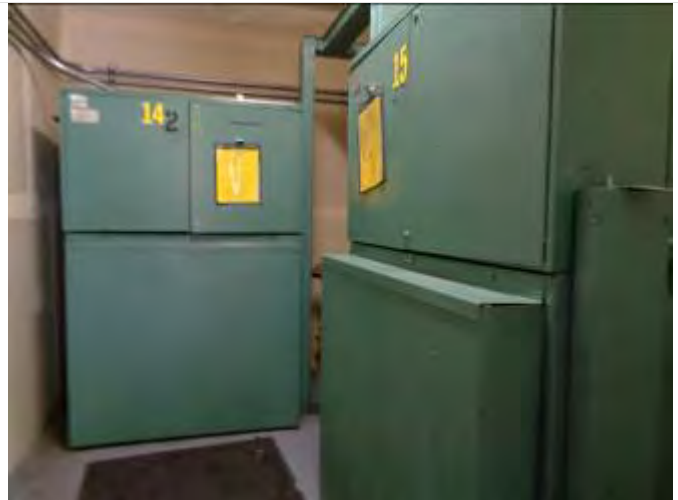
34. View of elevator equipment room – Building 2420
