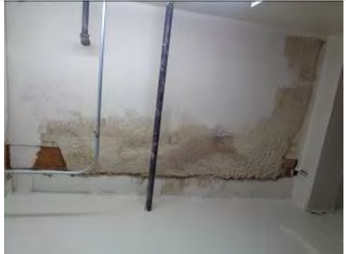
26. View of damaged drywall ceiling in elevator equipment room - Buildings 2400-2410
