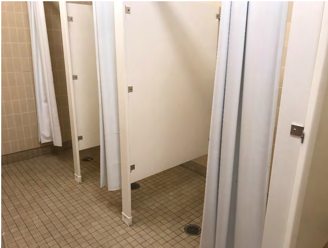
Photograph 21: View of shower drain in the bathroom of the Property.
