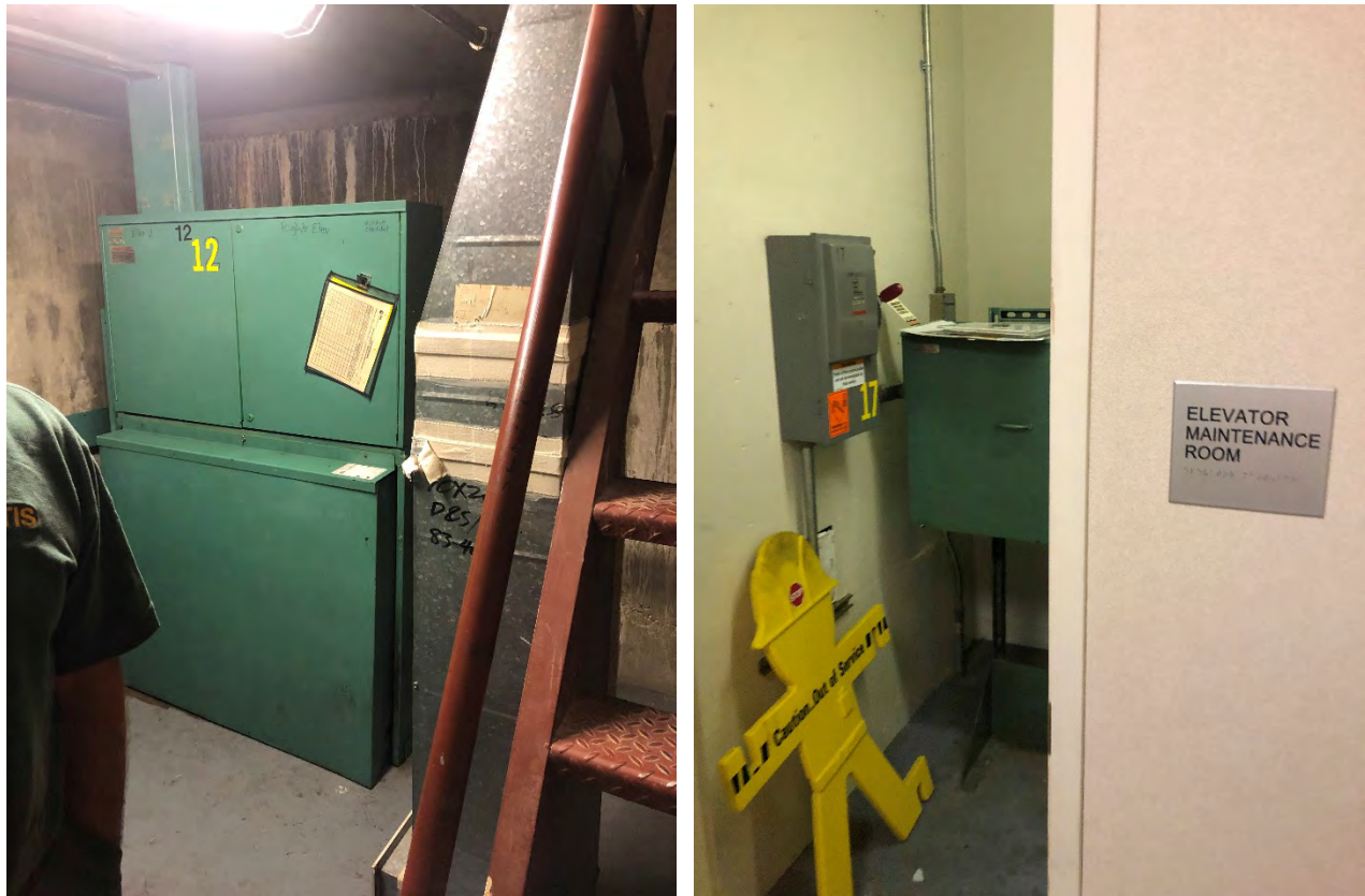
Photograph 9: Example of elevator equipment rooms.
