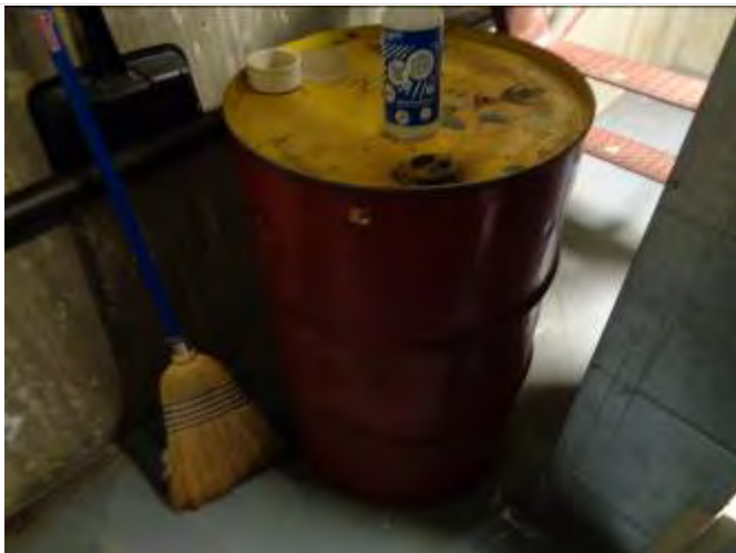
29. View of empty hydraulic oil drum in elevator equipment room – Building 2410
